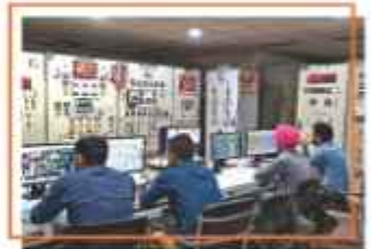
Boiler Control Room
