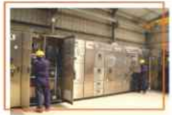
Electric Panel Manufacturing Bay
